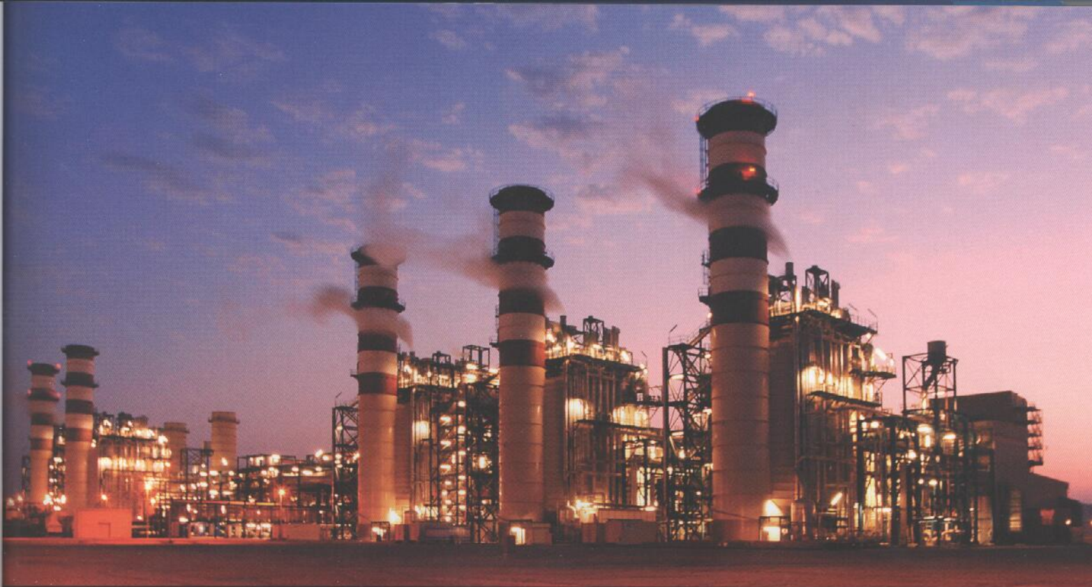
Oil refinery, Bahrain: the Kingdom was the first GCC nation to discover oil, in 1931
